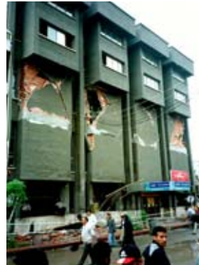
(b) In-plane failure
