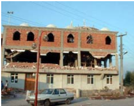
(a) Out-of-plane failure
