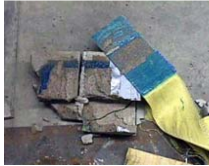
(f) Damage in the concrete blocks
