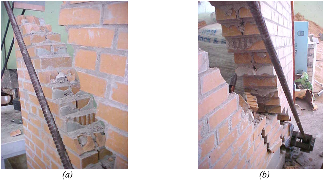
Fig.B.4 - 1. Splitting of clay units in wall CLW1
