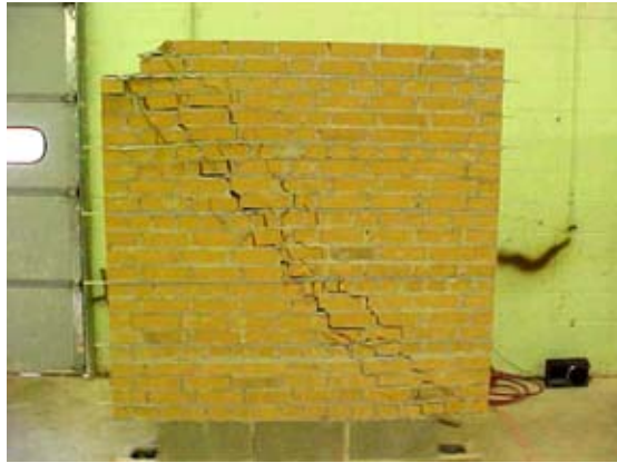
Fig. 6.13. Wall CLW2 after failure (front)
