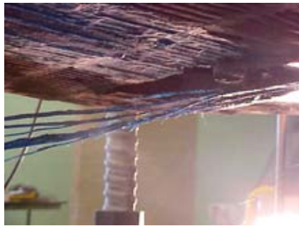
(e) BG3 – Fiber rupture + delam.
